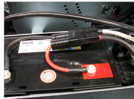
Fig. 41: Main cable battery
