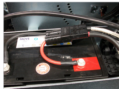
Fig. 41: Main cable battery
