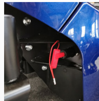
Fig. 83: Battery dicon. switch, inactive
